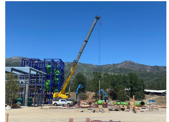
North Fork, CA – 2MW Electricity
