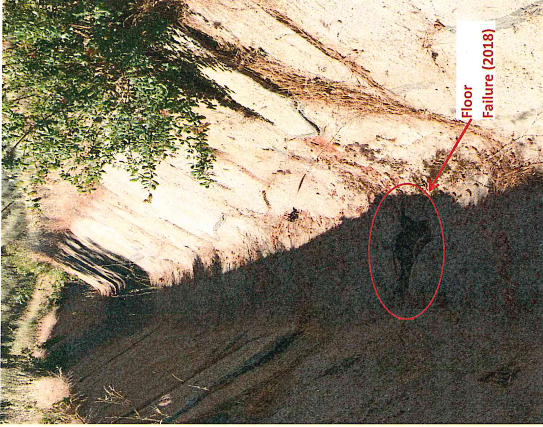
Figure 9 Lower Flume, Upper Section Floor Failure, 2018
