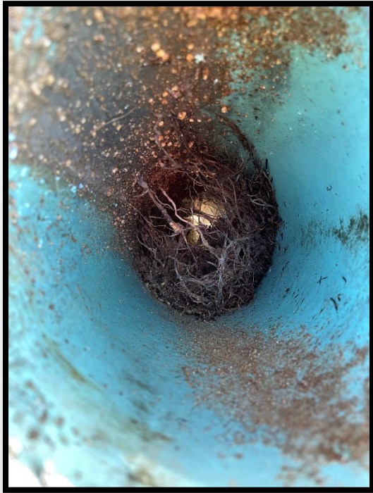
These roots were responsible for a Sanitary Sewer Overflow (SSO) into a nearby creek on Black Rd in Big Oak Flat.
