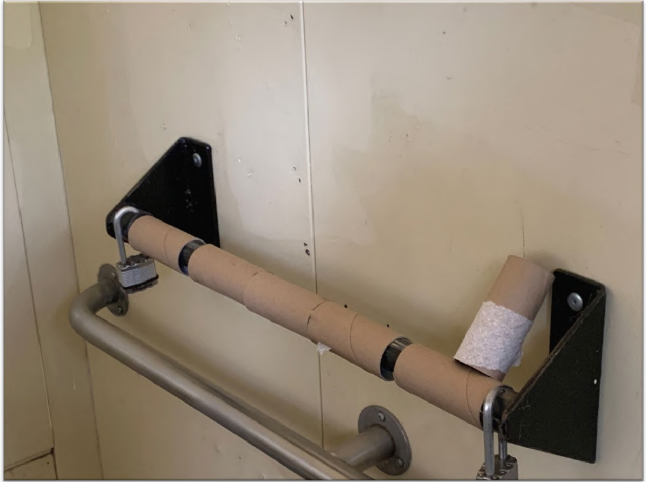
Figure 189: Mary Laveroni Park public restroom conditions.
