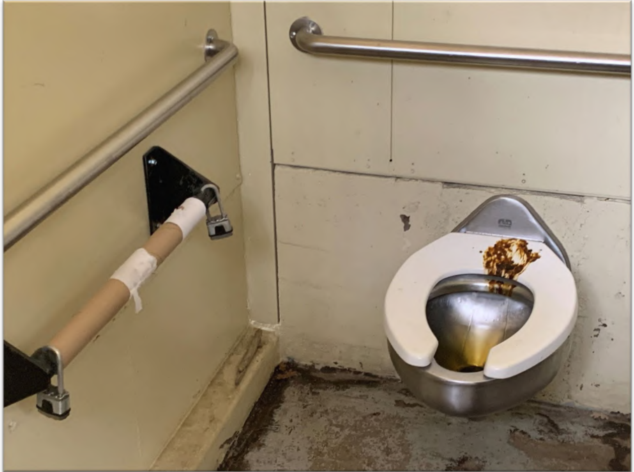
Figure 18: Project site A. Mary Laveroni Park public restroom conditions.
