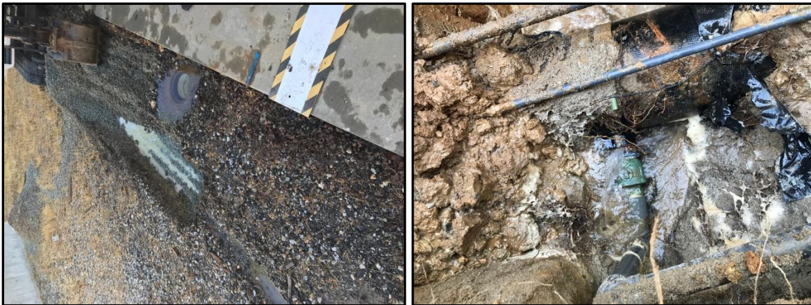
2G sample line leak at corporation stop
