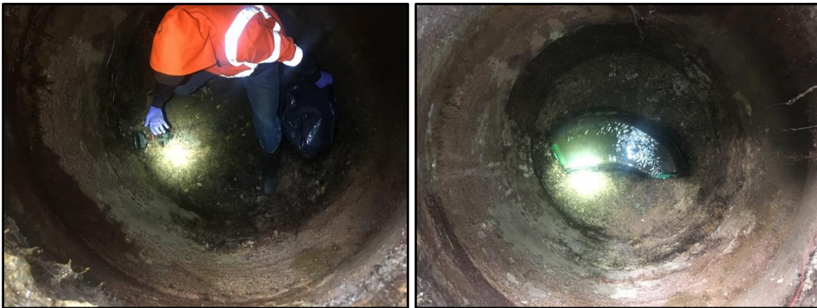
Partially clogged manhole found during inspections
