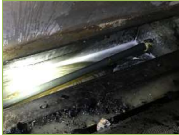
Broken airline caused by debris
