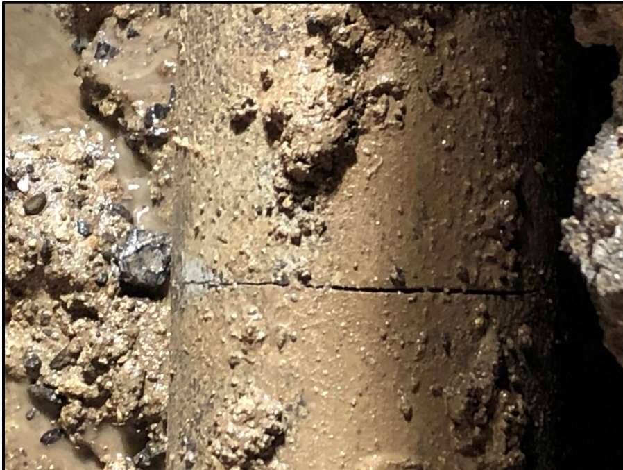
Broken 6" AC main line
