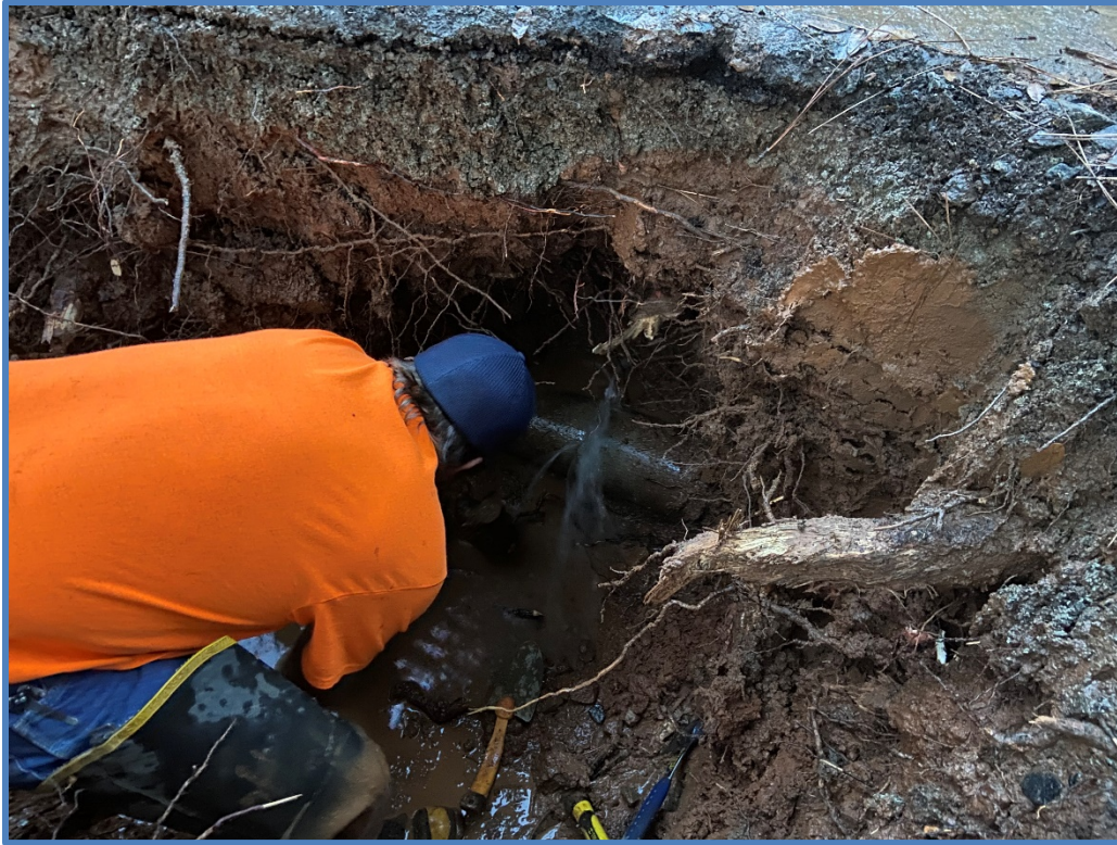
Roots around pipe broke the 6" Ac Main Line
