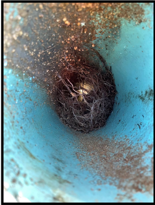
These roots were responsible for a Sanitary Sewer Overflow (SSO) into a nearby creek on Black Rd in Big Oak Flat.
