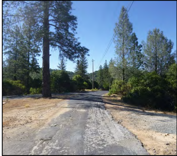
Photo 2. View SE, new water main route at intersection of Big Oak Flat Rd & Longfellow Rd,
