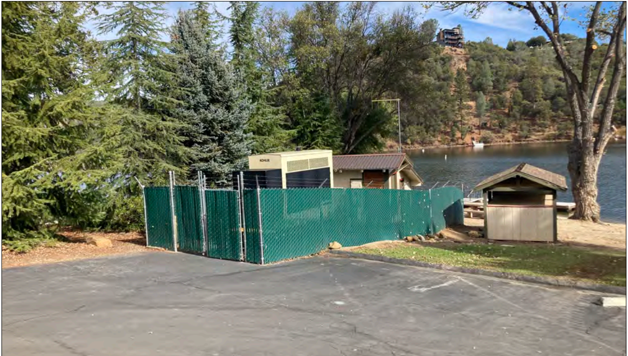
Figure 15. Photograph of the alternate water supply intake, facing northeast, showing urban land cover and Pine Mountain Lake.
