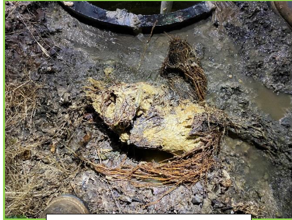
Root that was removed to restore flow
