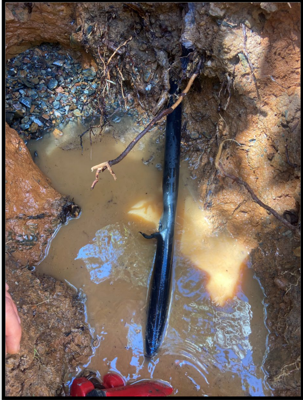
Leak caused by a contractor who was boring next to our line. It was marked out by us for their USA.
