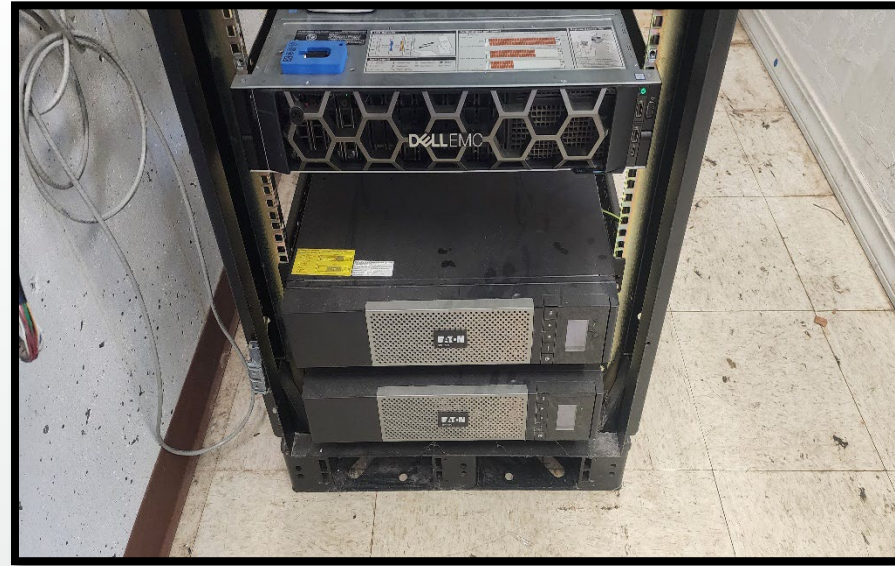
Dell Server & Backup
