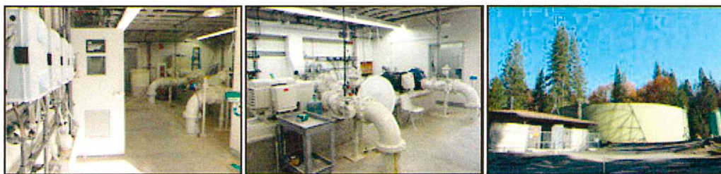
Big Creek Water Treatment Plant
